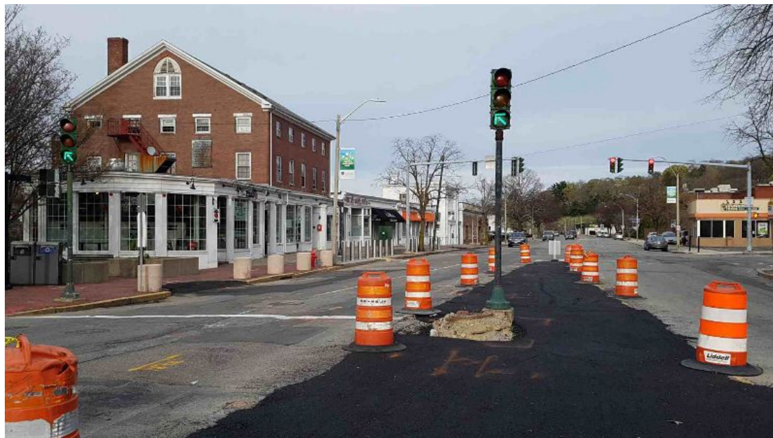
The Davis Tavern, seen at left with West Newton Square Enhancement Construction underway, is thankfully now landmarked, by a unanimous 5-0 vote of the Newton
